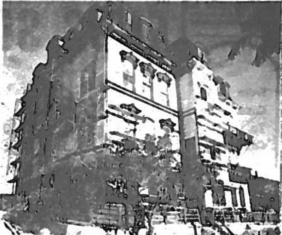
BACK SIDE of the Fourth Ward School, from the "D" street angle, reveals the fine restoration job on this section. The scaffolding indicates new work to be done will be on the south end.
