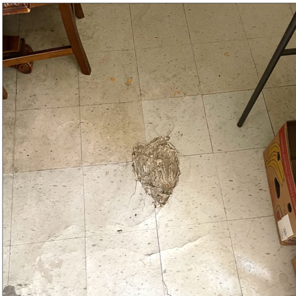
Damaged kitchen tile.
