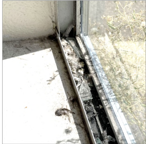
Broken glass in a windowsill.
