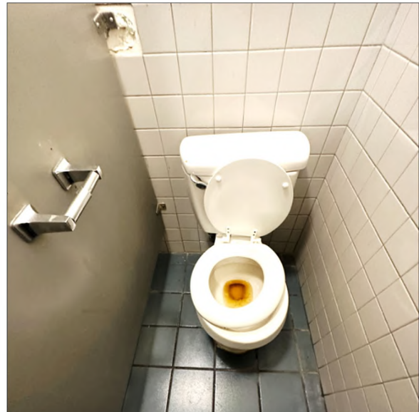
Unsanitary conditions in the bathroom.
