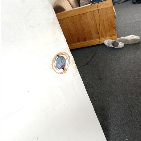
Child's door missing a doorknob.
