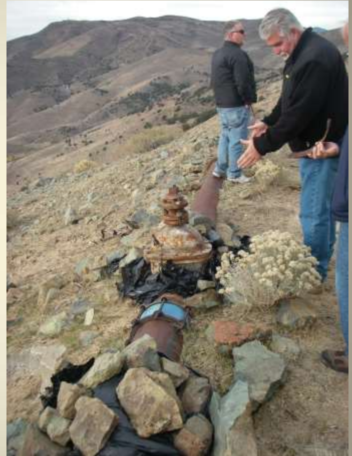
Gate Valve (5-Mile to V.C.)
