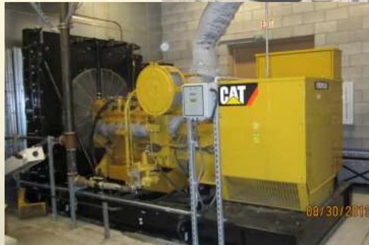
Marlette Generator and Generator Building
