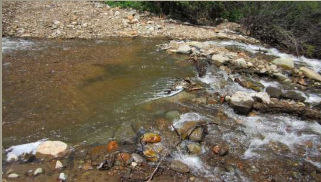
Inlet Flooded from Runoff
