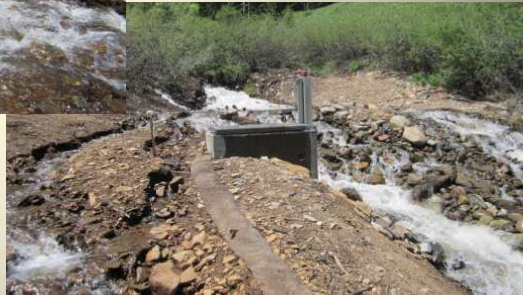
Sediment Trap Showing Runoff Bypassing Catchment
