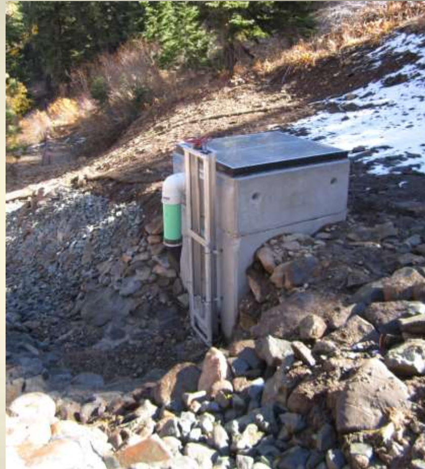
Sediment Trap with Extension/Overflow Piping and Reworked Drainage Channel
